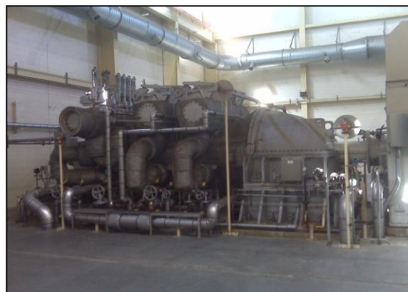
Steam turbine generator
