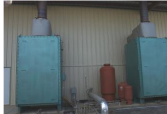
Cain exhaust heat recovery equipment
