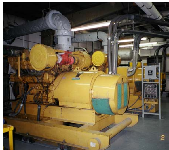
Figure 1: Angoon Power Plant
